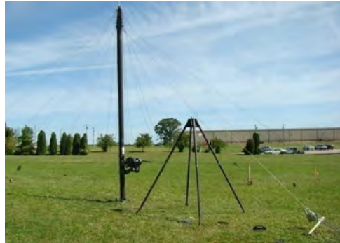
Figure 5-9 Position Gin Pole in Place with Its Center 3 Feet from Base of Mast
